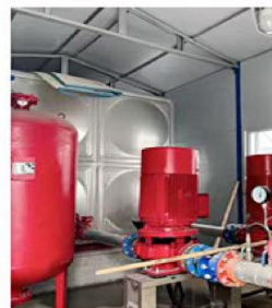
Fire water supply
